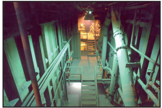
The combustion chambers of the Pittsfield Resource Recovery Facility can burn up to 240 tons of waste a day.
